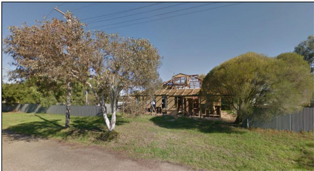
Above: The old hotel (2 nd location, portion 196) being demolished in May 2015. Courtesy Google Earth.
